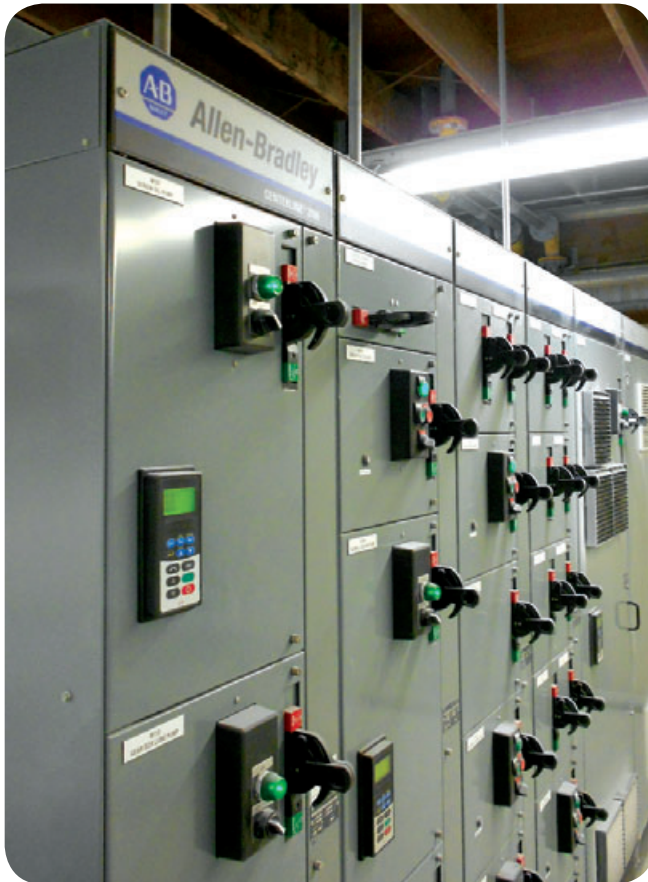
The MCC helps minimize facility downtime by quickly providing intelligent diagnostic information.
